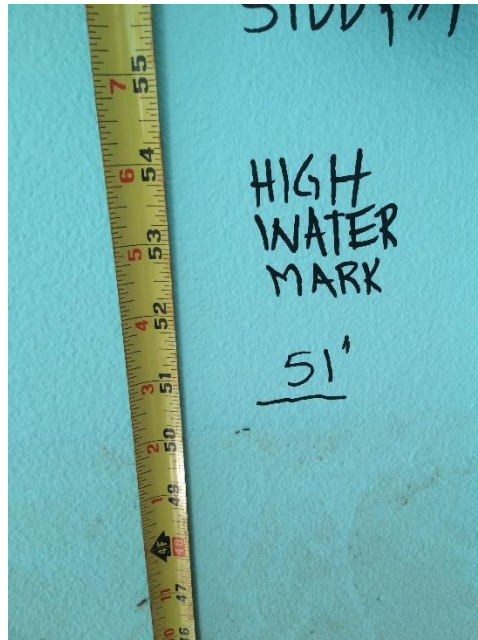
Figure 2 - Use a permanent marker to note the water height in each room. Photograph the mark along with a tape measure showing the height.
